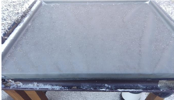
Roof with waterproofing PVC foil
